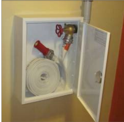
(A fire hose system cabinet)
