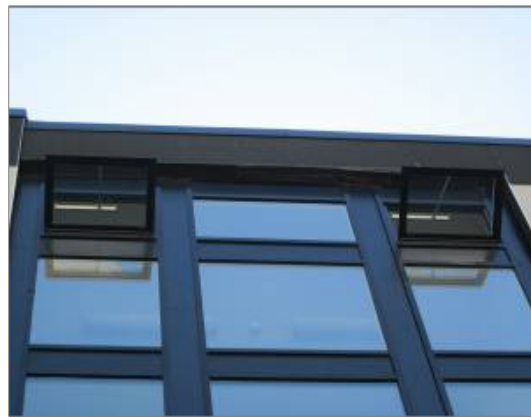
(stairway smoke vent)
