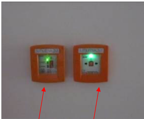
Opening vents (smoke removal activation buttons)
